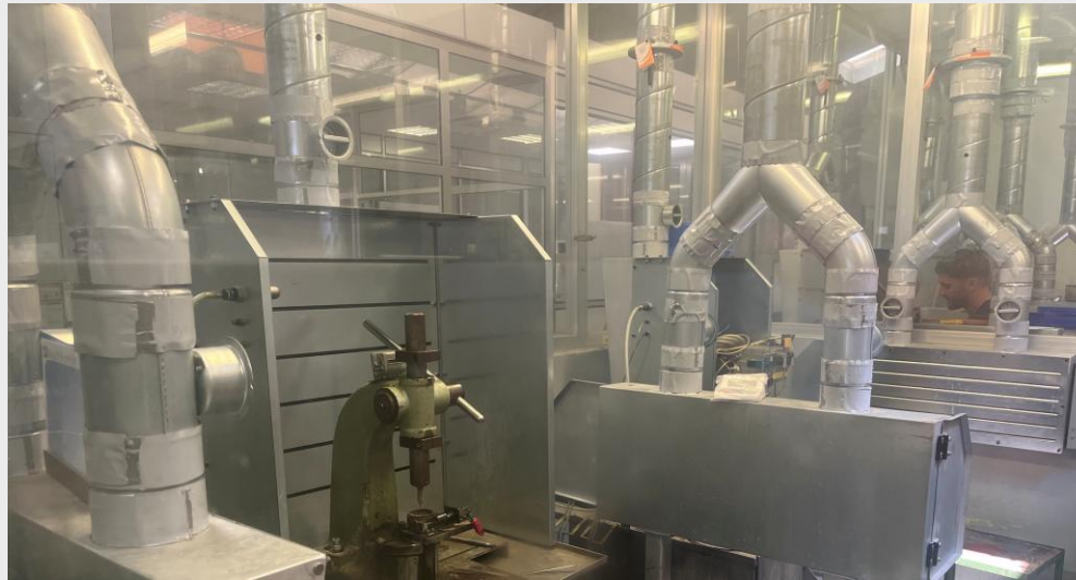
Fig. 17: New extraction system in Seltz
